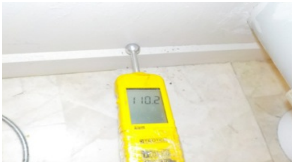
Figure 1: MINOR LEAK BEHIND TOILET, RECOMMEND FURTHER INVESTIGATION AND REPLACEMENT OF TOILET IF NECESSARY.
